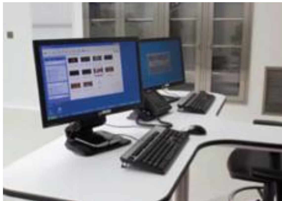
KVM over IP Controller along with Operator Management Solution
